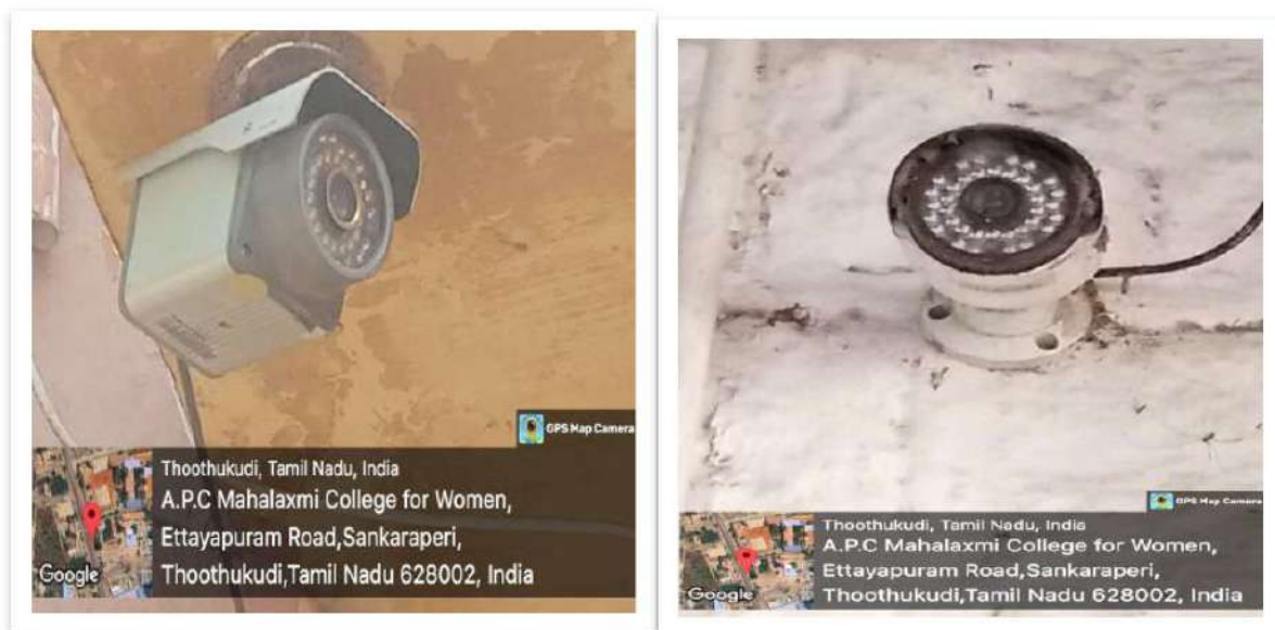
CCTV facilities within the campus
