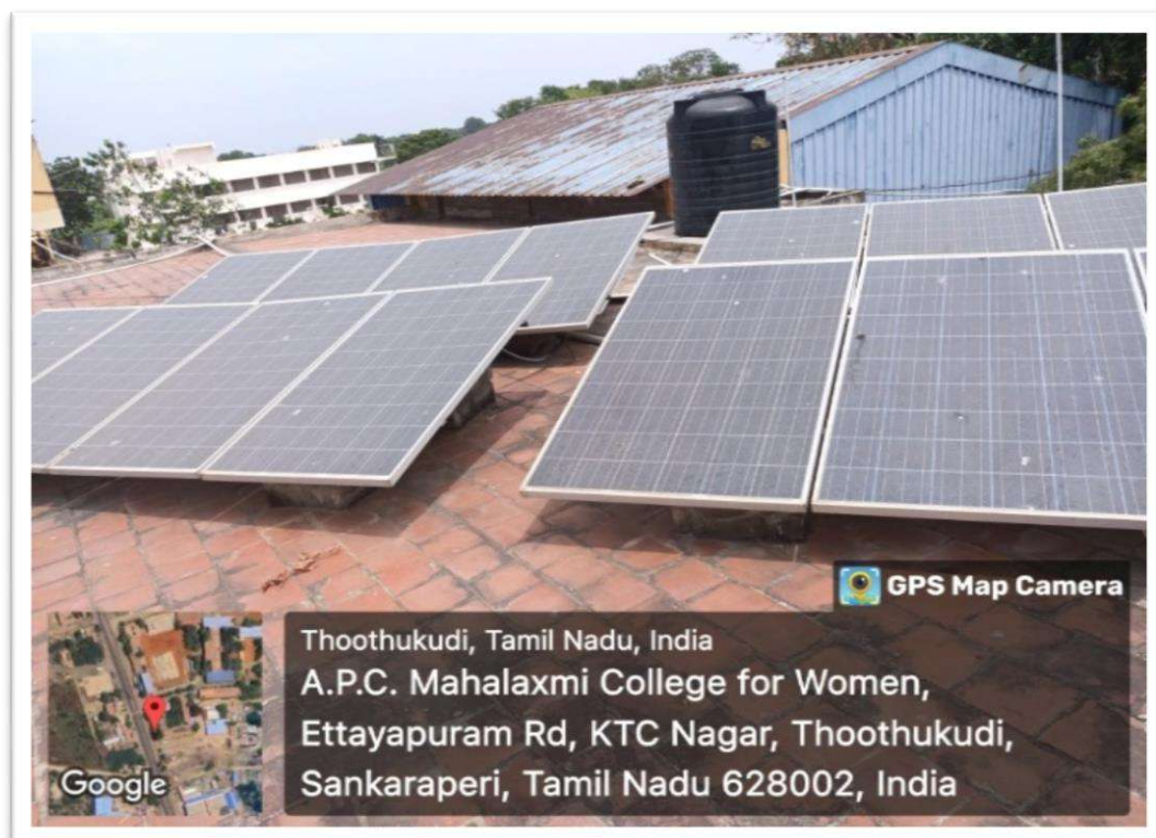
Solar unit at A.P.C.V Mahalaxmi Ammal block
