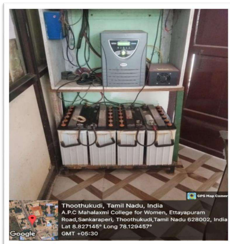
Distributing unit /Inverter
