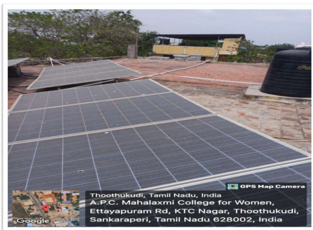
Solar units at Prof. A. Srinivasa Ragavan Memorial block
