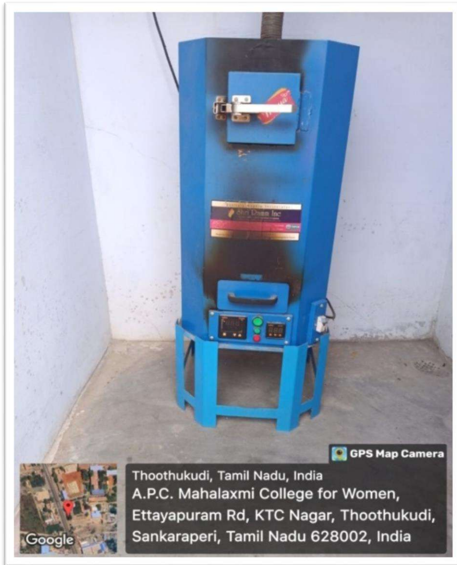
Incinerator at Srinivasan Ragavan block
